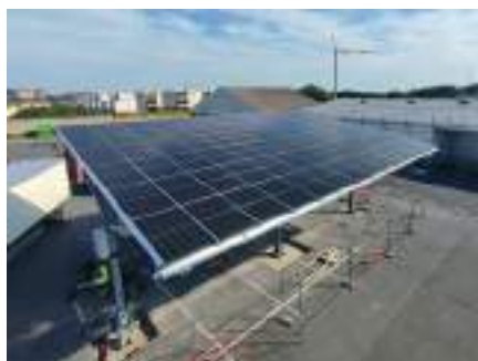
OMBRIÈRE PHOTOVOLTAÏQUE 36 KWC
